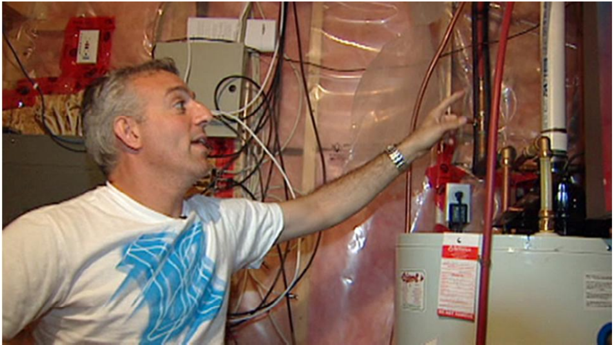
Frank Cappellino, a LaSalle, Ont., homeowner shows where a pipe burst, flooding his basement last fall. (Karen Brady/CBC)
