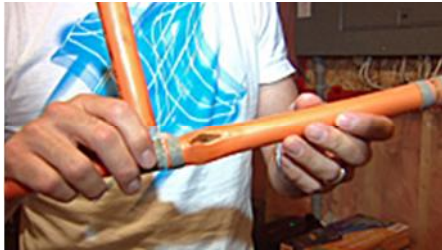
Cappellino shows the Kitec hot water pipe that burst last fall.
